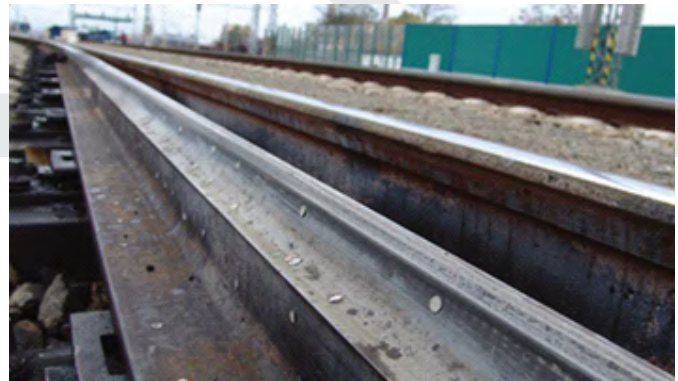
Switch rail with increased resistance in the track
